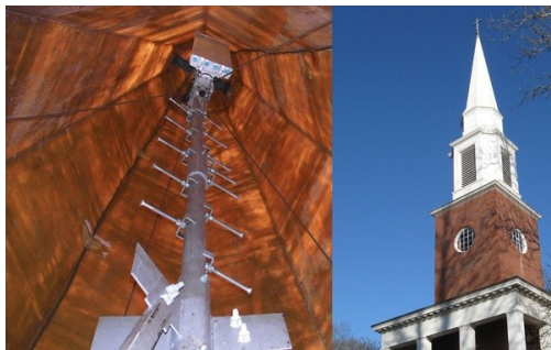
Inside a church steeple reveals a ladder providing technicians access to the cell antenna
